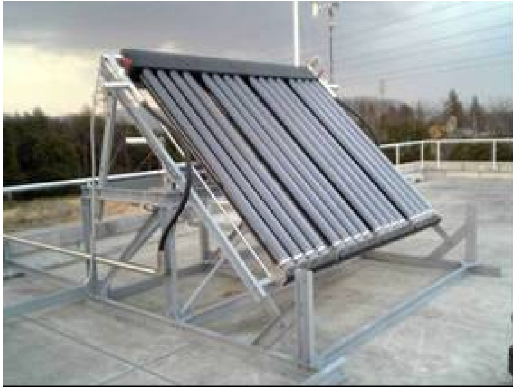
Solar Hot Water System
