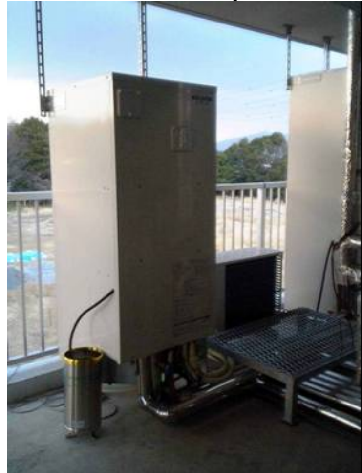
CO 2 heat pump Hot Water System
