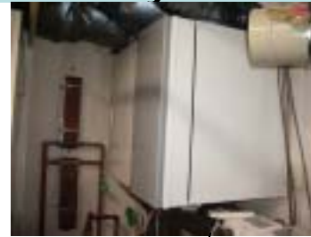
ventilation unit with a heat recovery element In a laundry room as an air chamber room
